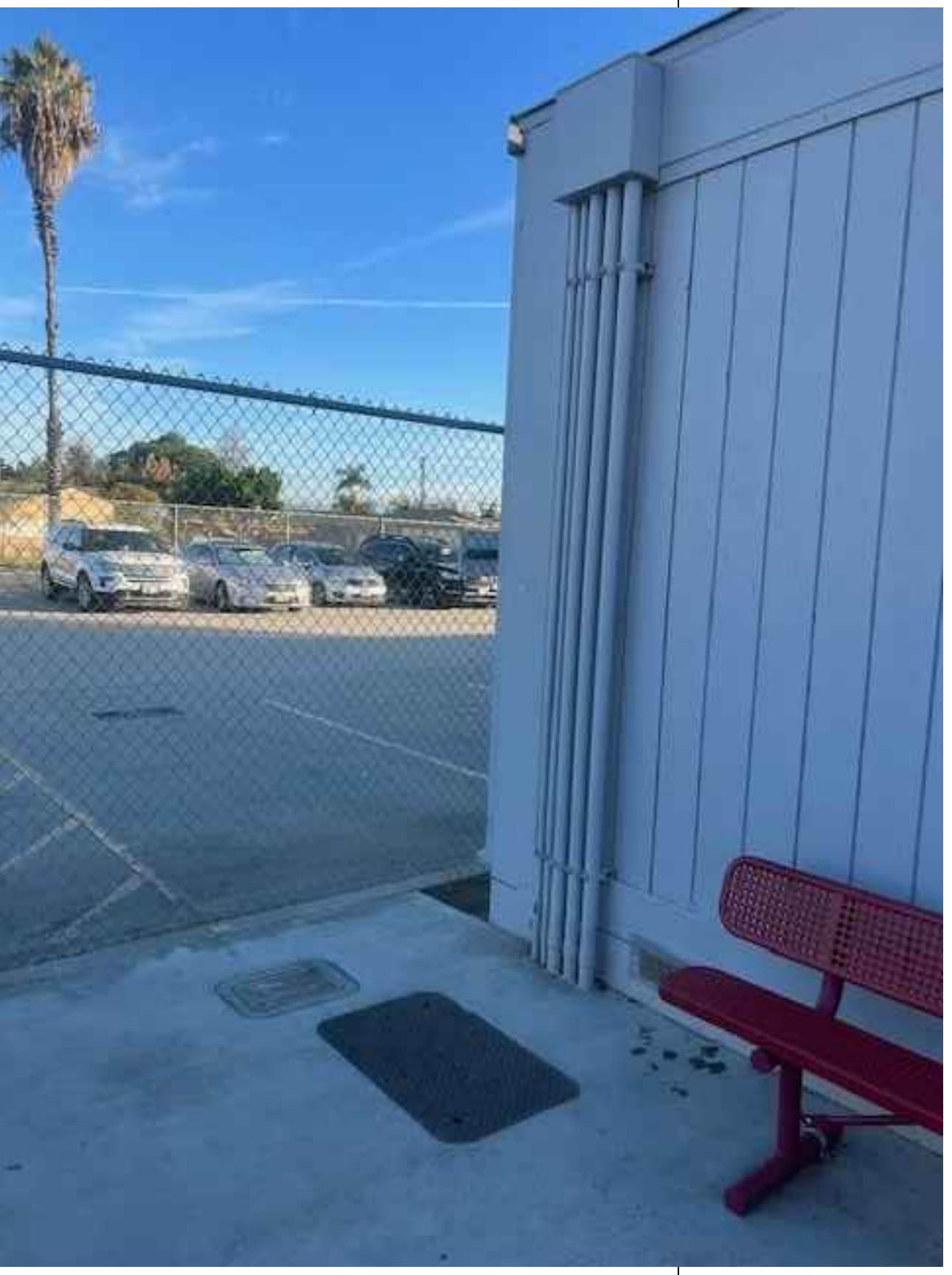
EXISTING CONDUIT RISER PICTURE ③
